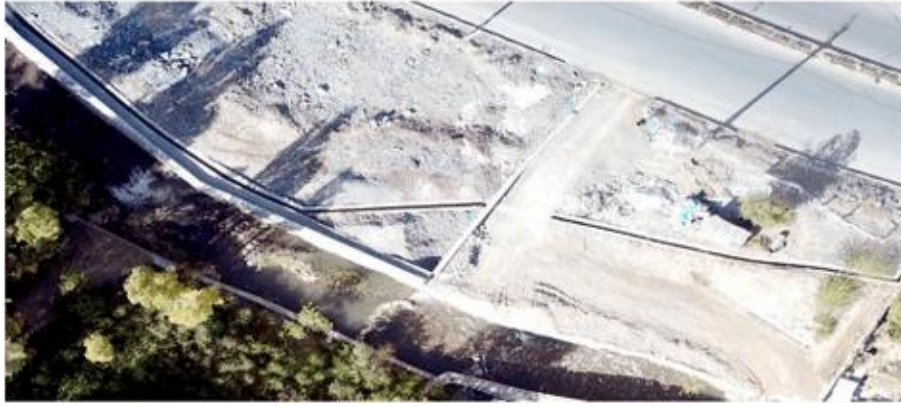
Figure 5. Existence of wooden barriers inside the canal and steep slope of the riverbank.
