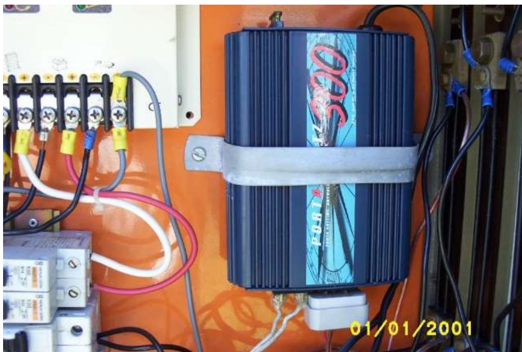
FIGURE 9 – Modified senoid tension inverter PWZ 300 installed in the system.
