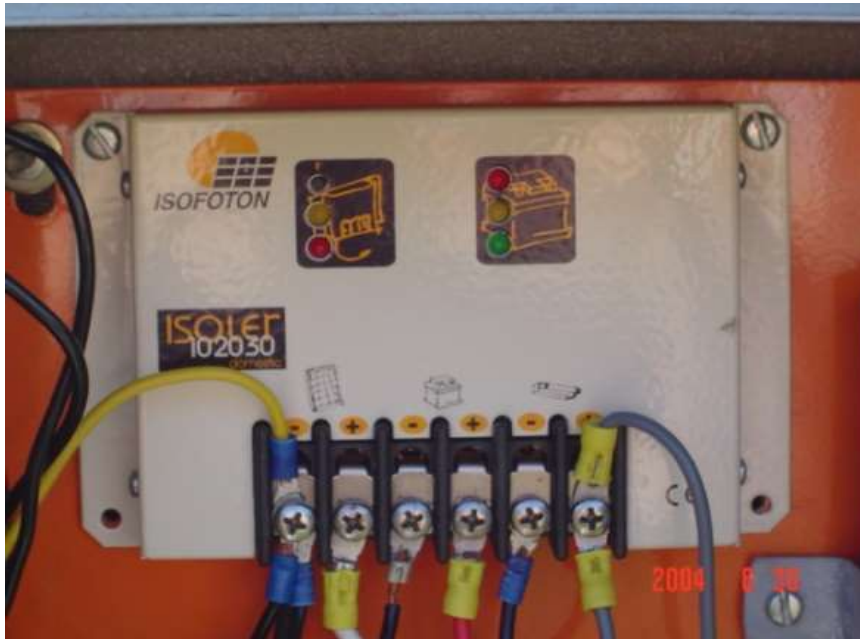
FIGURE 4 – Charge controller ISOLER connected to the photovoltaic panel, battery and charges.
